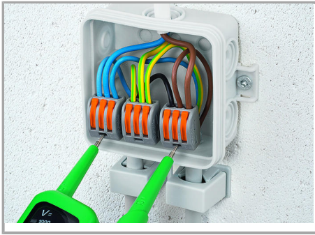
Testing via Profi-LED+ voltage tester (206-806).
