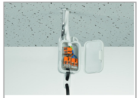
Pendant light connection in suspended ceilings
